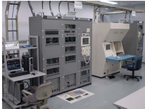
Communication control system
